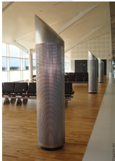
ABOVE Displacement ventilation totems have been installed at Birmingham Airport in the UK
